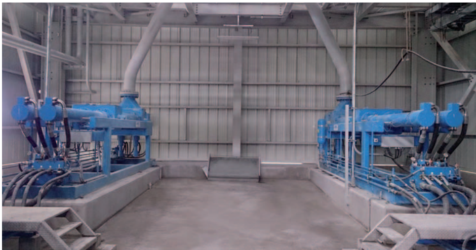
2 ABEL Solids Handling Pumps for backfilling of mine tailings mixed with cement
