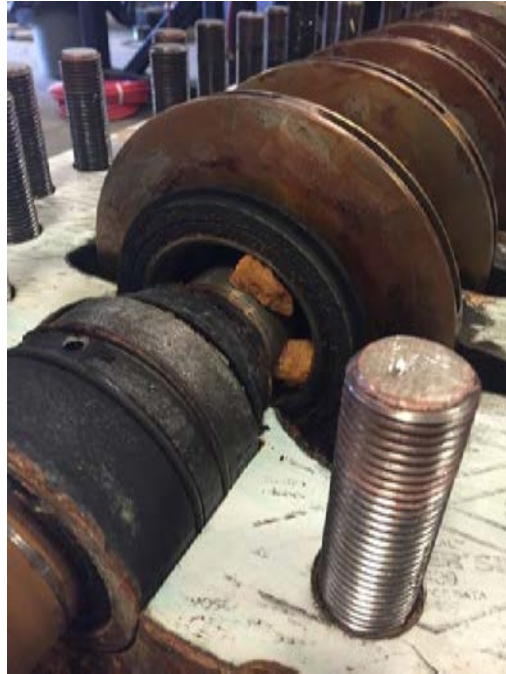
Debris in 1 ST stage suction impeller
