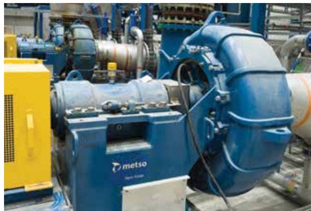
Horizontal slurry pumps
