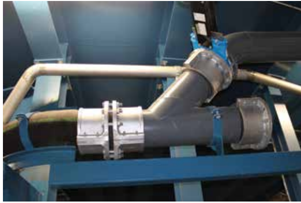
Branch pipes and valves
